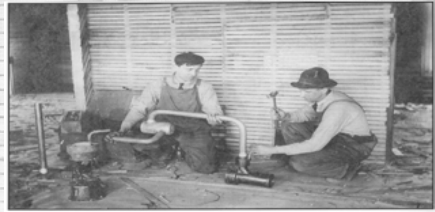
This photograph which was taken on the job in 1909, shows Local 157 Apprentice Henry Zimmerman (left) watching intently as Local Union journeyman Plumber Herman Holthaus (right) demonstrates the correct way to make connections on sections of lead pipe.
