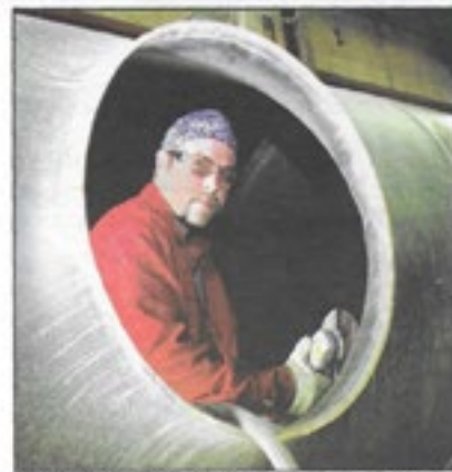
The winning Photo was from the November 2007 issue. It showed Local 157's Dustin Roberts inside a large diameter pipe at the Freitag-Weinhardt shops in Terre Haute.
